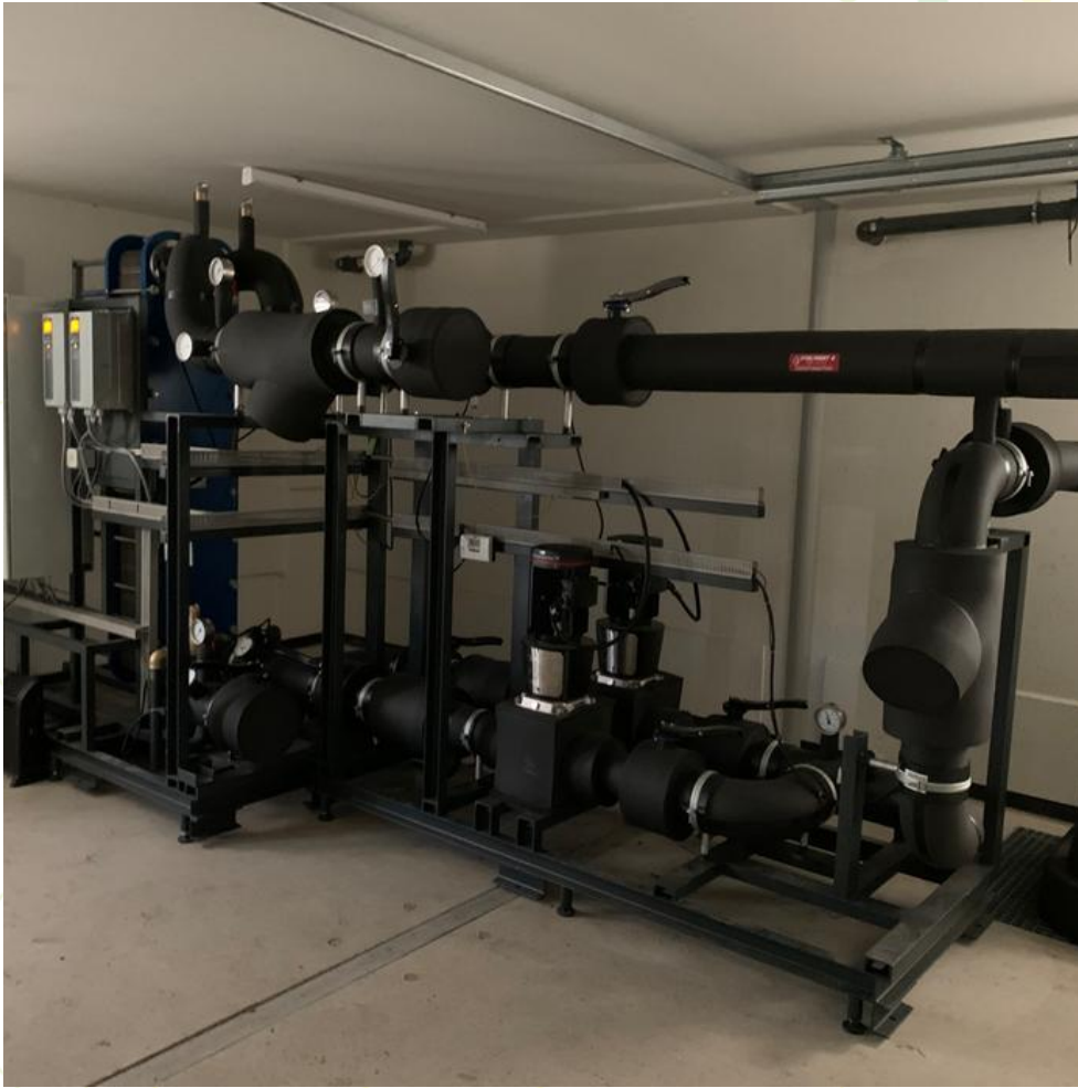
Figure 8: the heat exchanger
