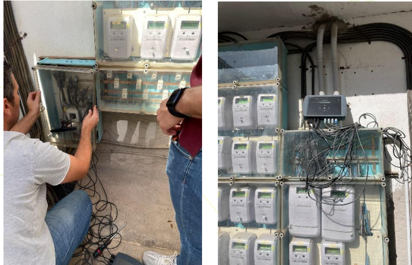
Figure5. Installation of network analyzers
